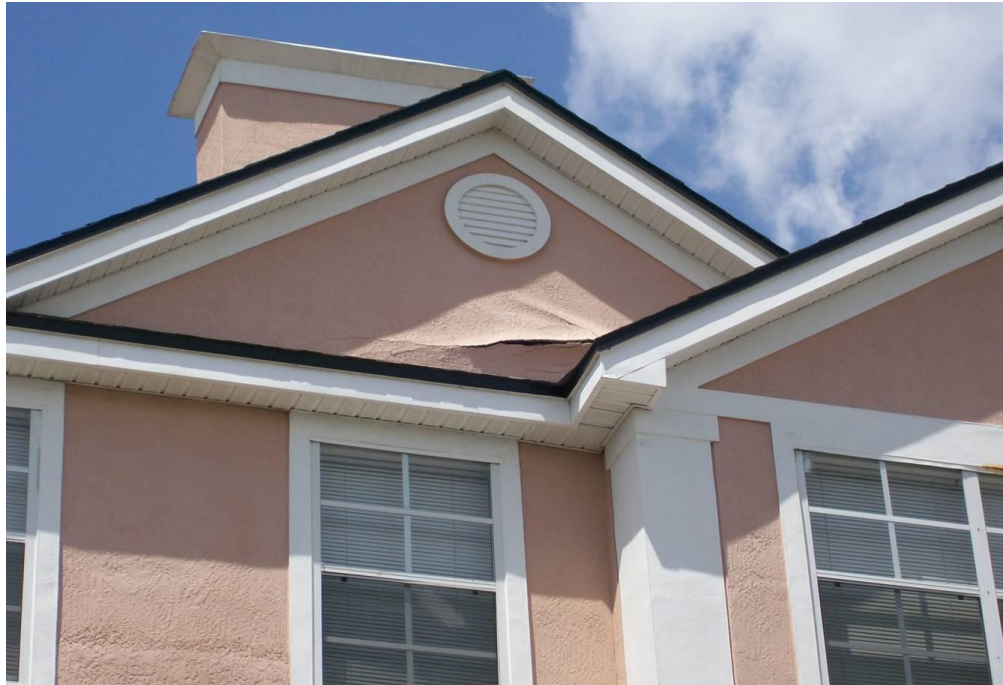
Photo #4 – Stucco detaching from building.
