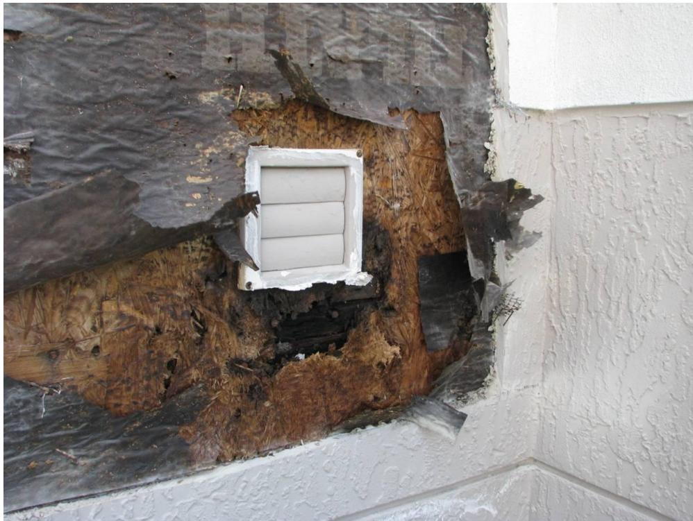
Photo #3 – Decay damage at un-flashed dryer vent.
